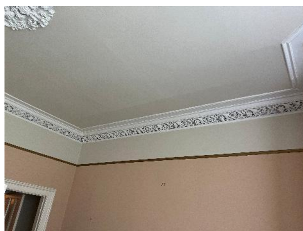
Uneven ceiling (lounge)
