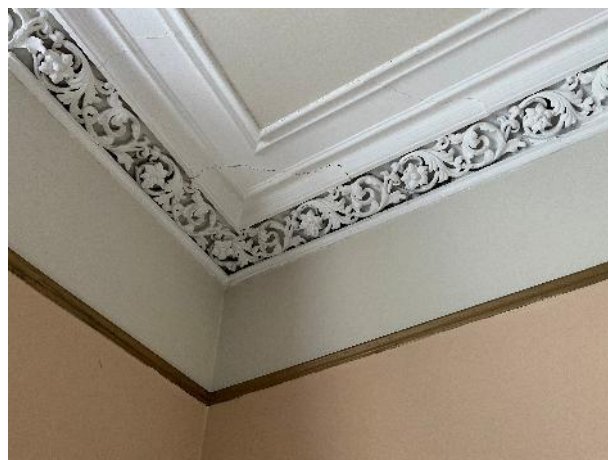
Crack in cornice within lounge
