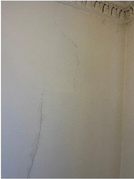
Crack in bedroom wall (gable)
