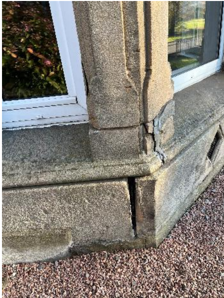
Movement in bay window and historic repair
