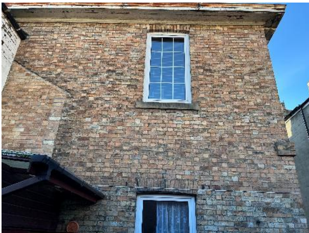
Minor crack above bedroom window
